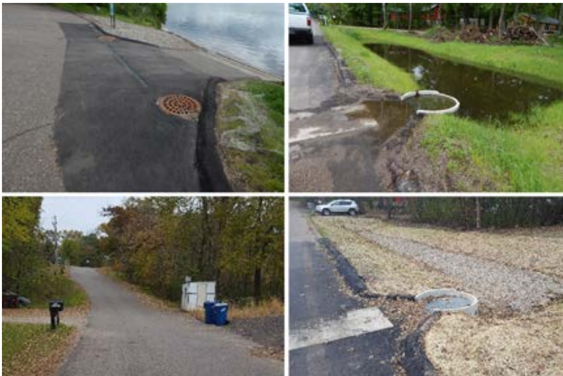
Photos: 224th Ave infiltration basin capturing and treating local stormwater (2017). Slotted drain at boat landing, which captures runoff from street and parking area.
