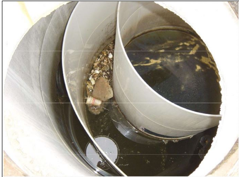
Coffee Shop Hydroguard Removing Trash, Oil and TSS
